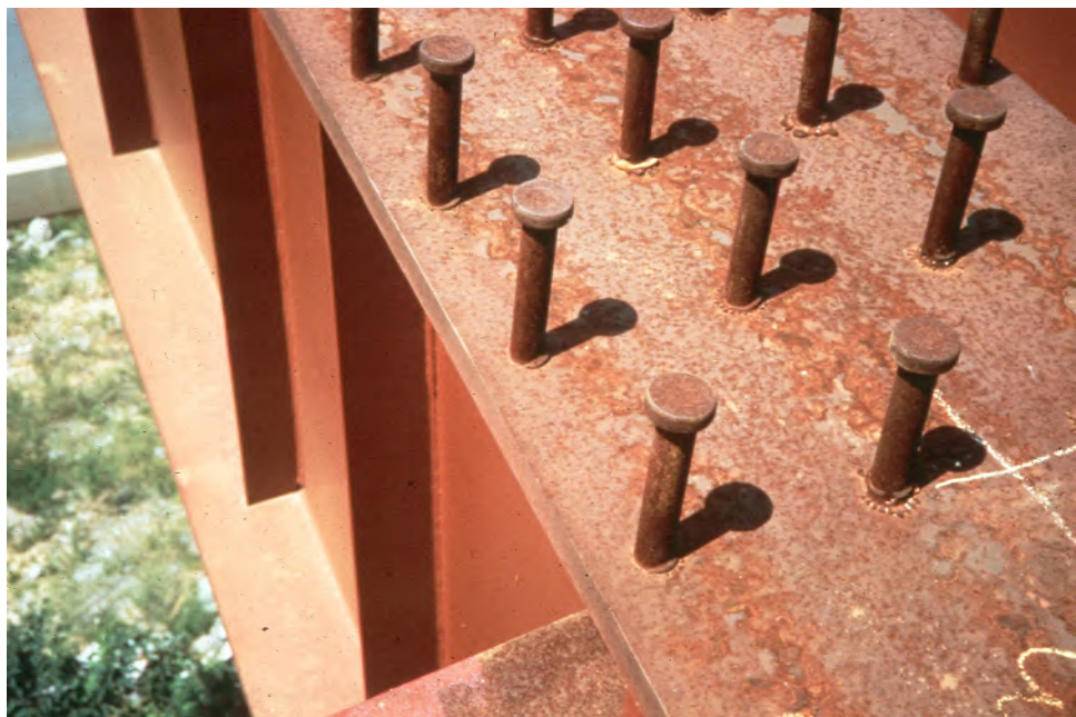
Figure 3.1.31 Shear Studs on Top Flange of Girder (before Concrete Deck is Placed)
