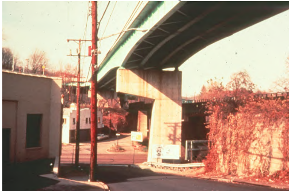
Figure 3.1.6 Unusual Concrete Shapes
