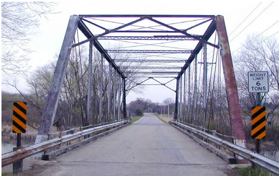
Figure 3.1.41 Weight Limit Sign and Object Marker Signs Lighting
